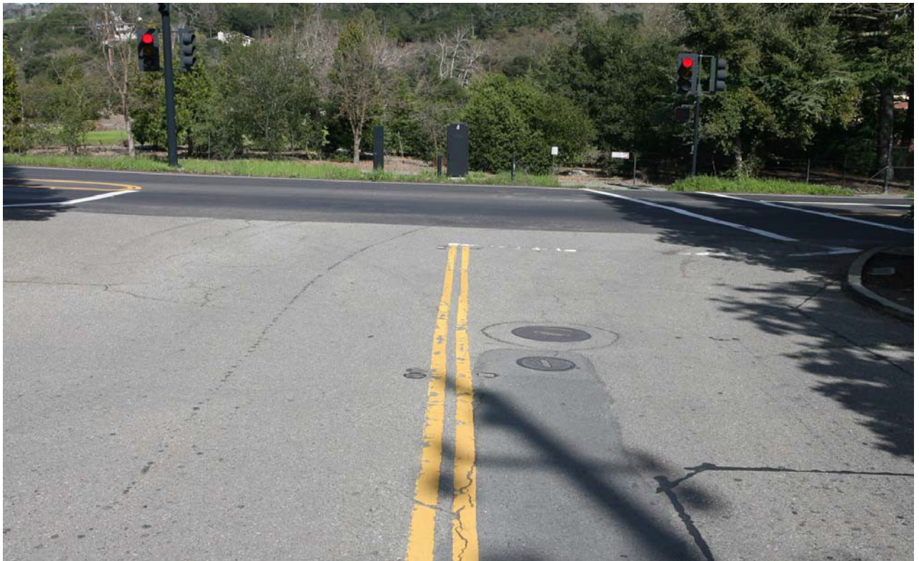
Claremont Avenue PCI 80
